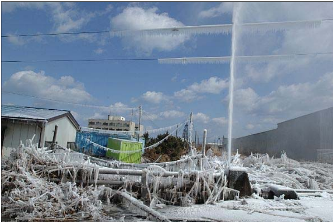
Figure 5.A Damaged Water Pipe Shoots into the Air, Hachinohe, Japan
